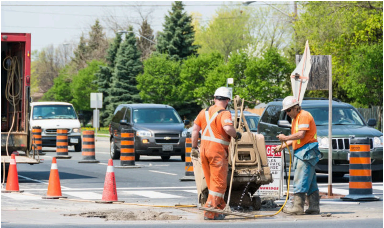
ROBERTO MACHADO NOA VIA GETTY IMAGES Two workers do repair work on a Toronto roadway.
